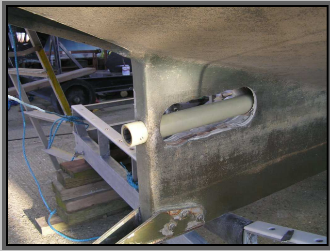
Above: Stern tube in place in skeg prior to being epoxied in place. A 22mm drive shaft is being used.
